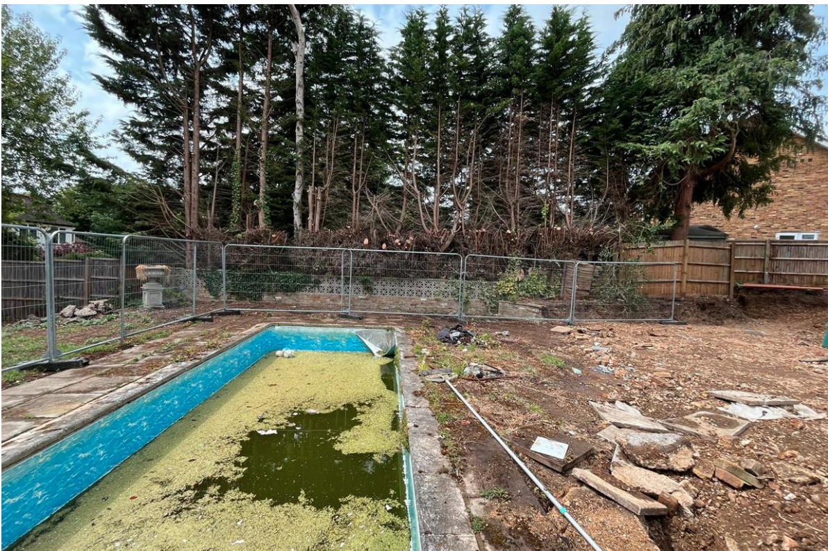
Protective fencing in place on boundary with No. 22 and to rear garden / no equipment on site
